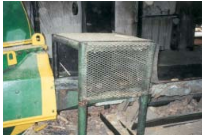
Fig. 1: Protective cage over chipper infeed
